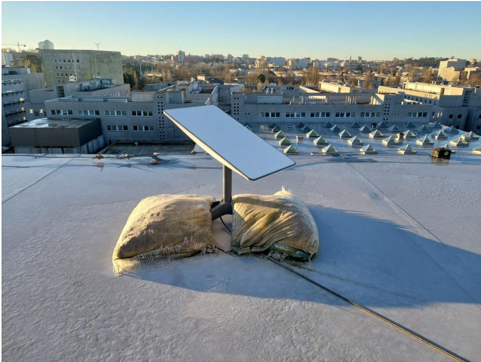
Figure 9. Antena of the Starlink system installed on the rooftop of INESC TEC's building, in Porto.
